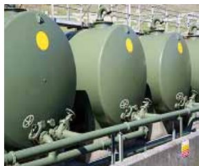
Storage tanks inside a concrete bund.
